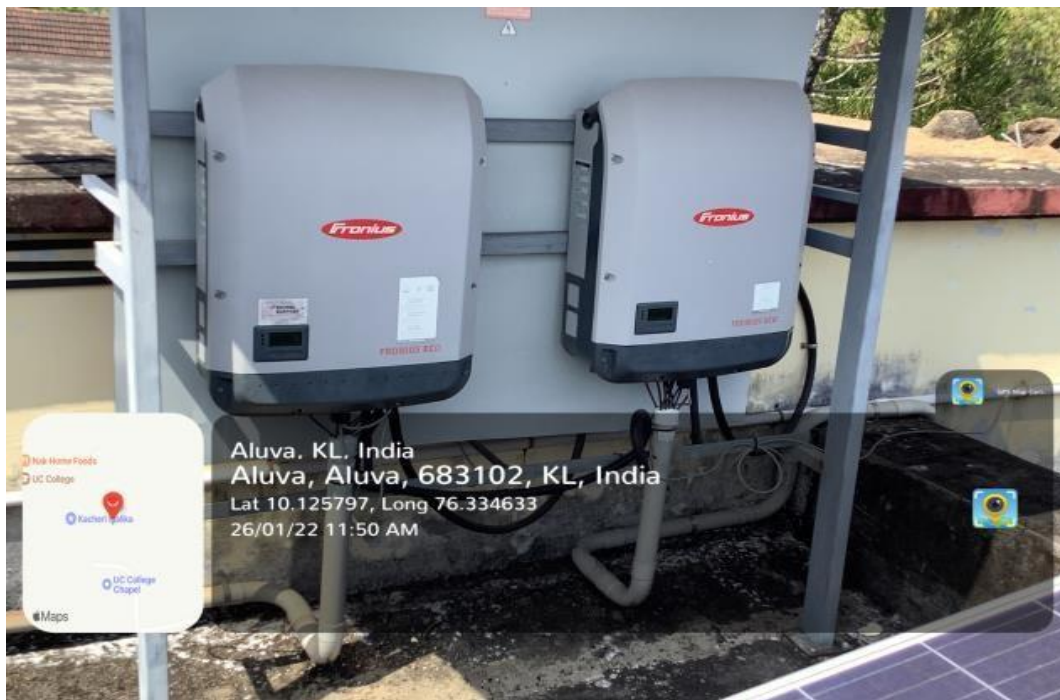
Figure 3 : Solar Grid Inverter
